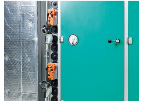
Damper actuators on air handling unit
